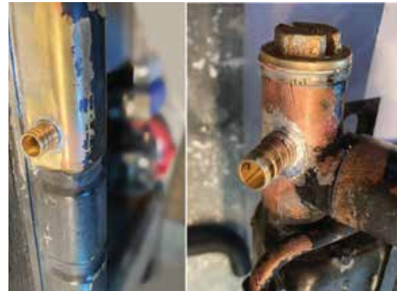
Header tank take off
